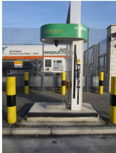
HYDROGEN FUELING STATION
