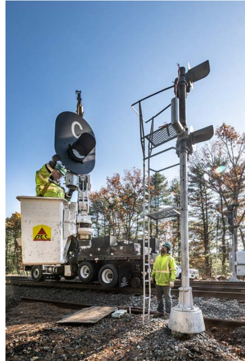
As part of a federal mandate passed by Congress in 2008, the MBTA is installing Positive Train Control (PTC) technology across all commuter rail lines.
