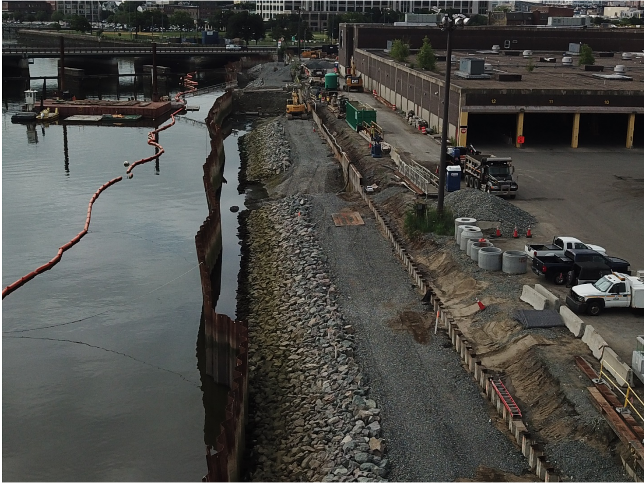
An aerial view of the Charlestown seawall, which protects more than $140 million of MBTA assets at the abutting bus facility.
