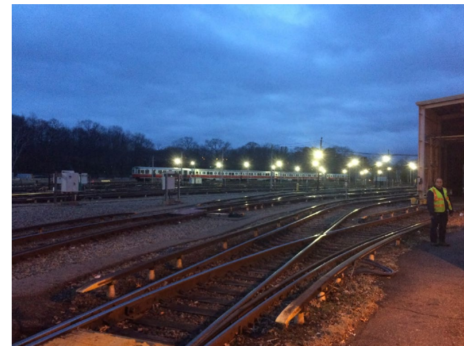
Existing Yard Lighting
