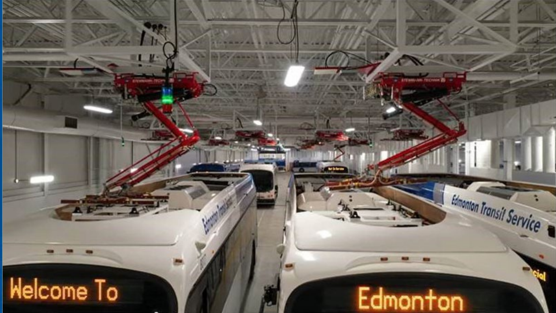
Edmonton Transit Service (ETS) battery electric buses charging by overhead pantograph charger.
