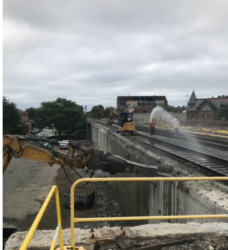
Granite Stone Removed and Demo at Laraway Lot with dust control (August 2022)
