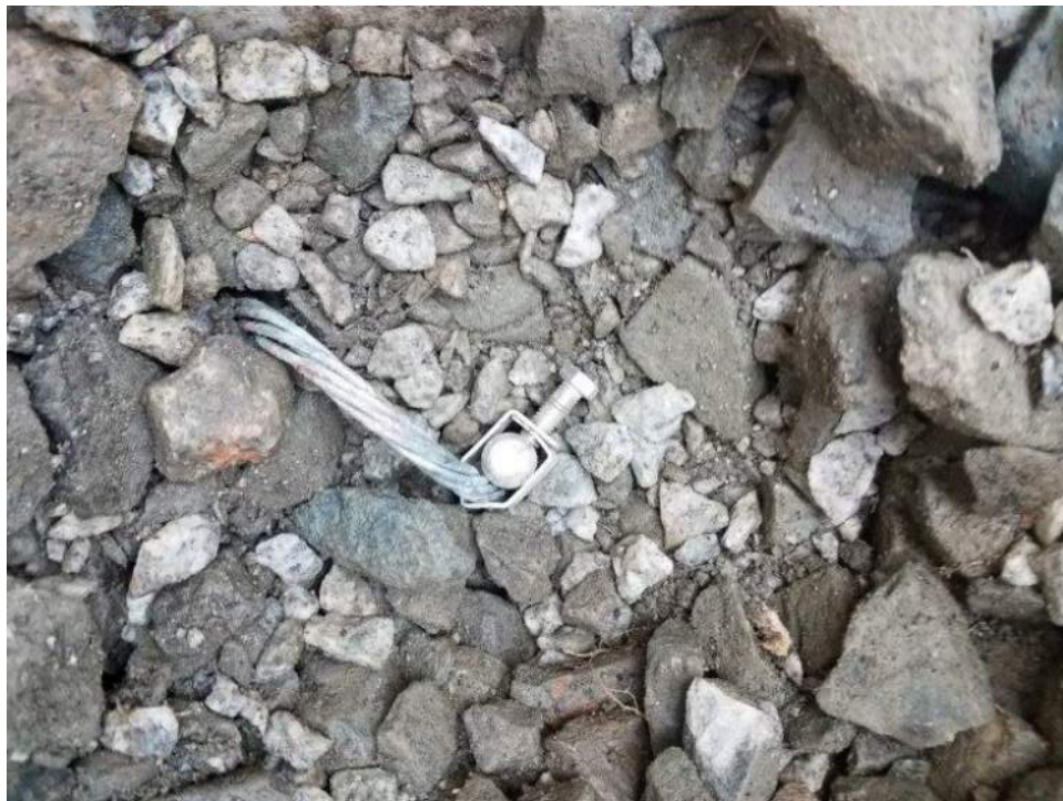
Photo 4. 3/4-inch SS grounding electrode.
