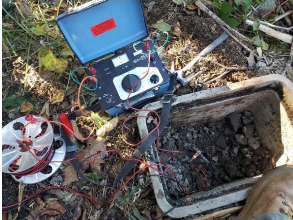
Photo 9. Grounding electrode resistance testing.
