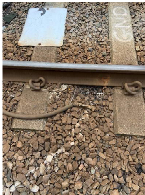
CADWELD – GROUND RETURN
