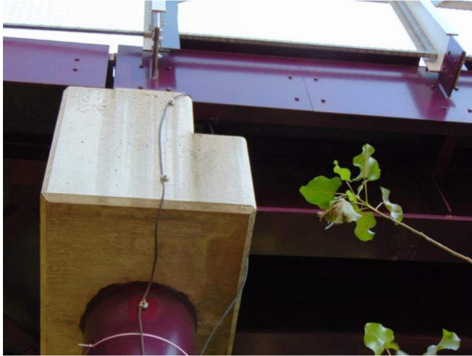
Photo 3. Grounding conductor 1/0 AWG. Pier 24 Northside
