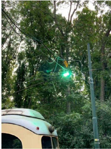
Trolley #3268 passing the Catenary cutout switch
