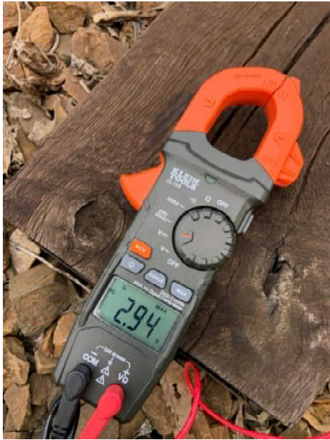
Stray Voltage Measurement (Outbound of Station Track to Fence)
