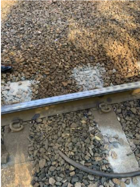
Discoloration Outbound of Station
