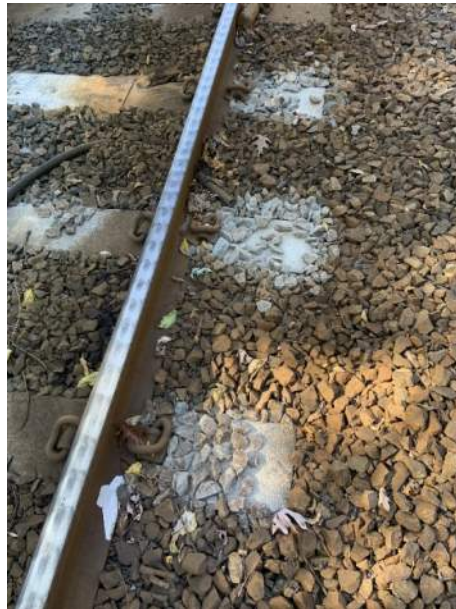
Discoloration Outbound of Station
