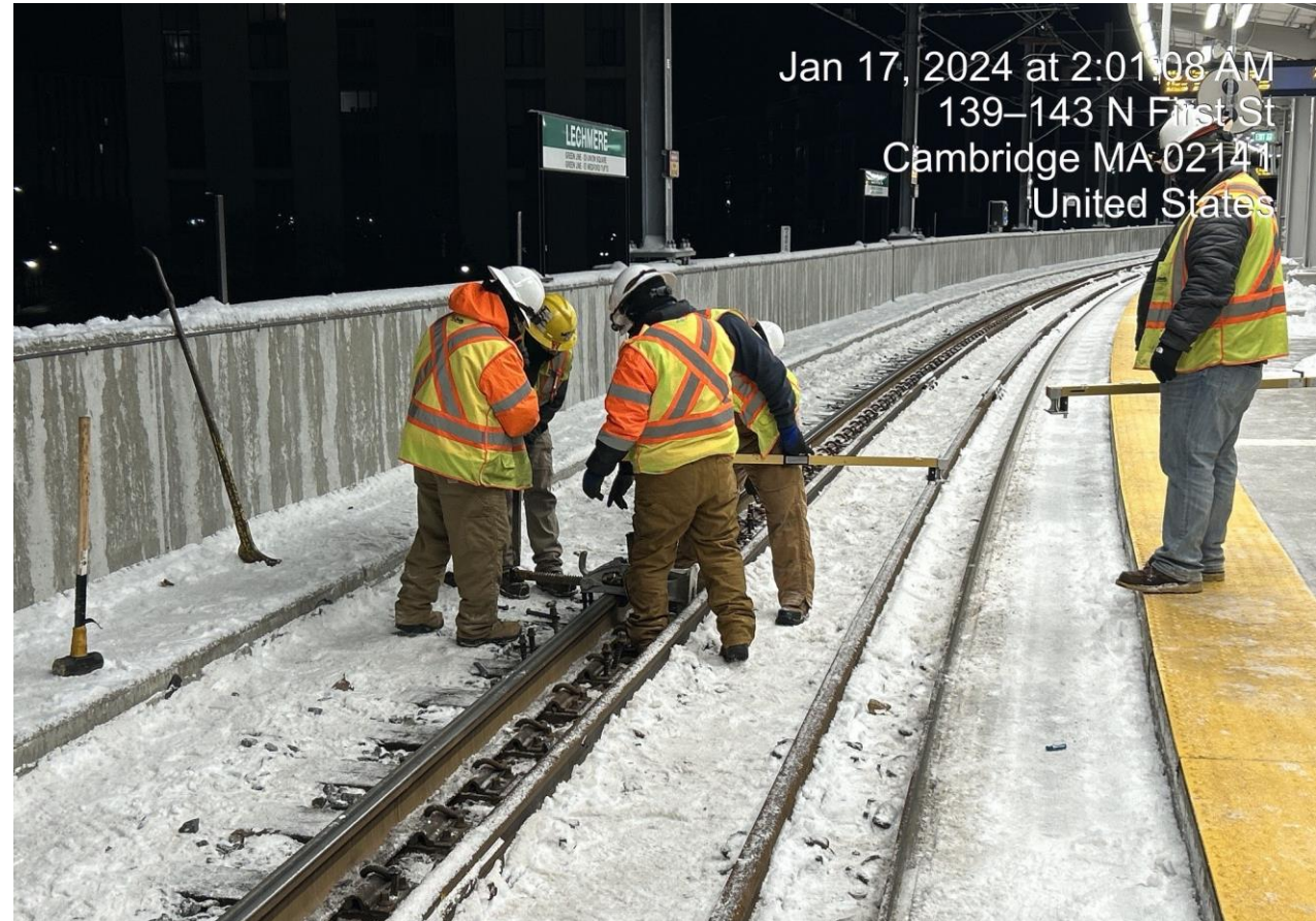
Hand re-gauging a short section of track that was out of tolerance
