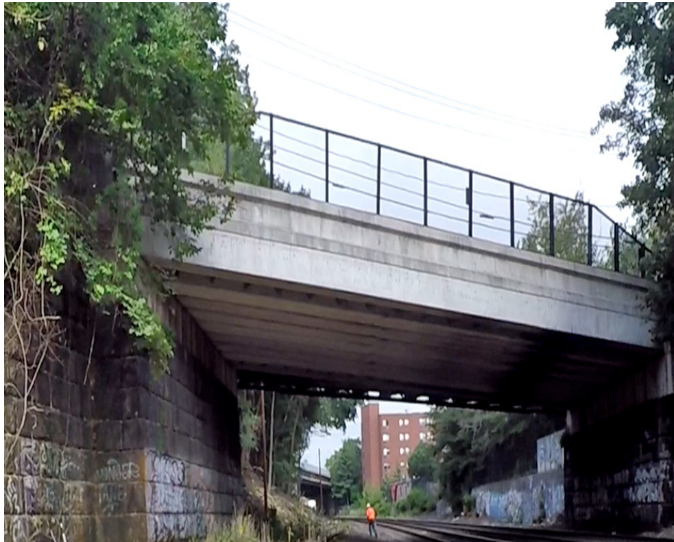
Figure A5.2.2-9: An east elevation (looking west) showing the existing Walnut Street Bridge. The GLP Community Path Elevation Increase ATC significantly reduces work at this location by having the path go up and over rather than tunneling underneath the street.
