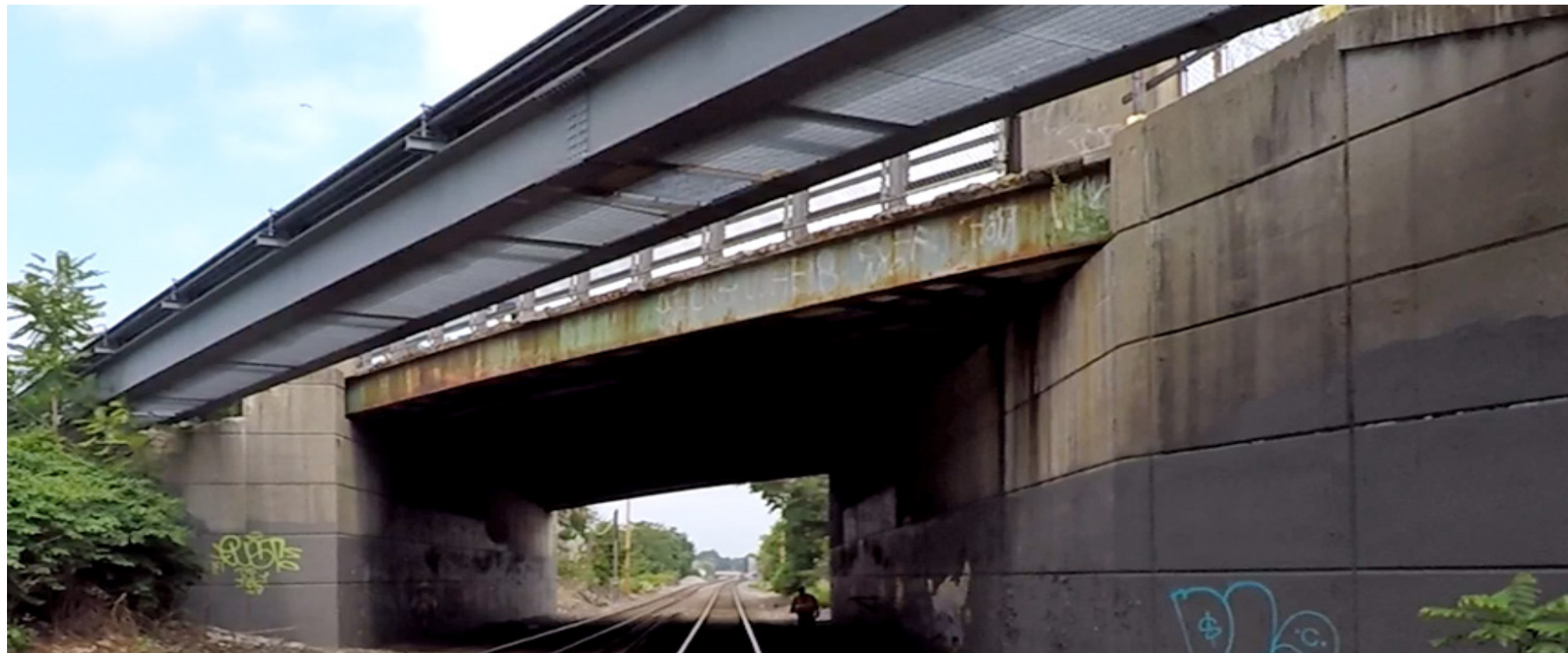
Figure A5.2.2-11: An east elevation (looking west) showing the existing Broadway Bridge. GLP will replace the existing bridge with a two-span continuous structure with a sufficiently long span to accommodate the two new GLX tracks as they diverge coming in to Ball Square Station.
