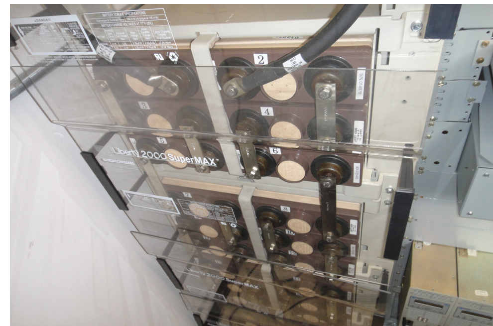
Figure A5.2.1-5: GLP will provide reliability through battery backup power to safeguard the integrity of the signaling system
