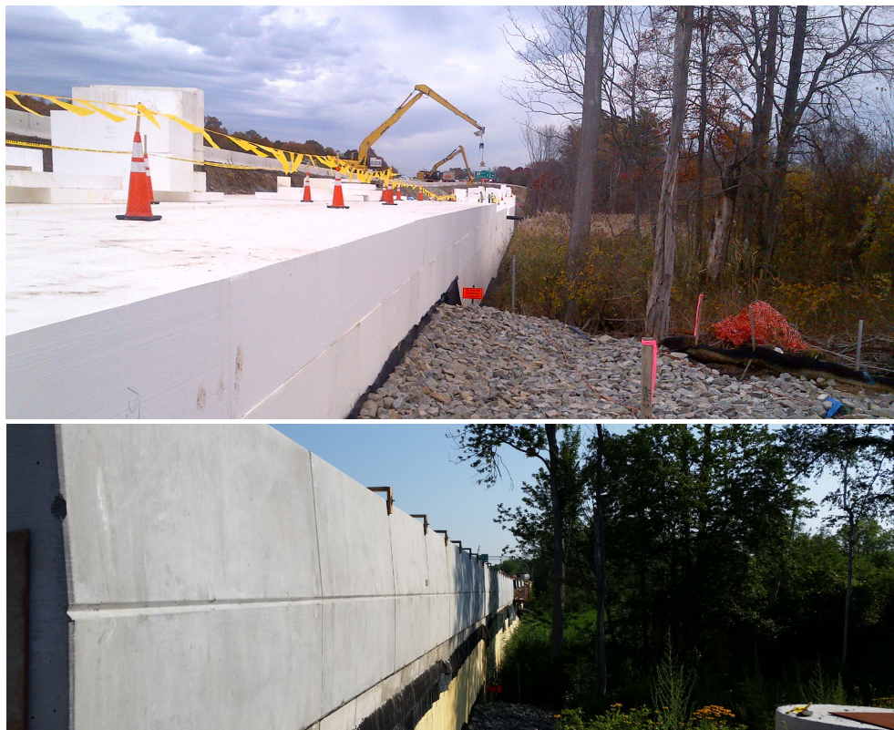
Figure A5.2.2-8: On the Whittier Bridge project, GLP designer WSP used EPS block to widen 2,000 feet of I-95 adjacent to wetlands, which aided construction in the existing ROW and accommodation of poorly consolidated soil.
