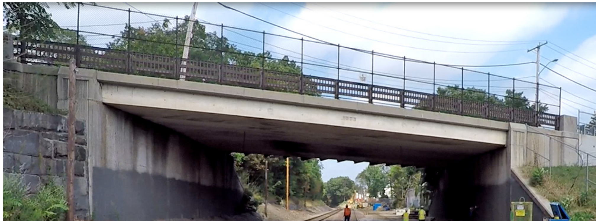
Figure A5.2.2-12: An east elevation (looking west) showing the existing College Avenue Bridge. GLP will maintain the existing bridge structure and remove a sidewalk to accommodate a new right-turn lane. We will also provide a new pedestrian bridge on the west side of the bridge to provide pedestrian access from the west side of the alignment on Boston Avenue, near the new College Avenue Station to the east side of the alignment on College Avenue.
