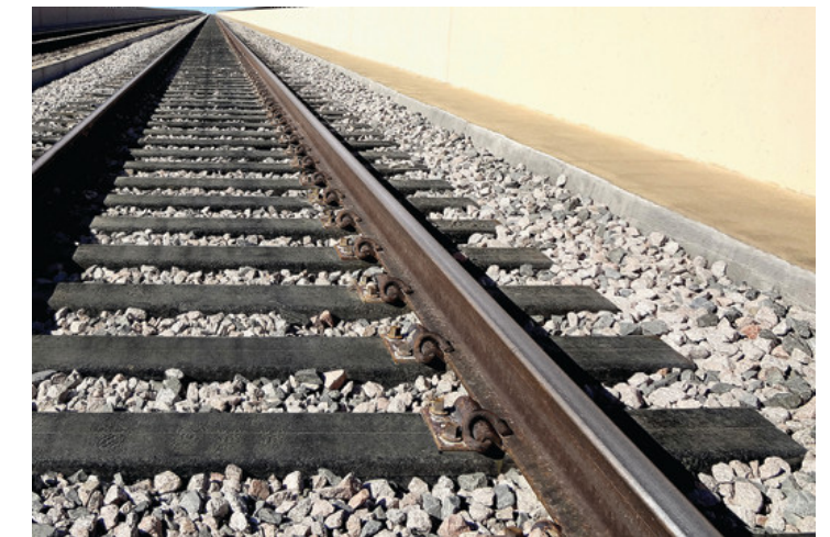
Figure 4.1-15 Typical 1-inch ballast-to-rail separation WBG will use to reduce stray current on the GLX Project.
