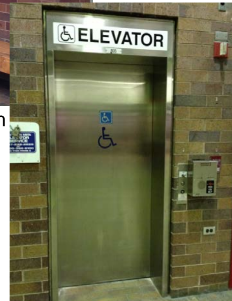
Platform Elevator 805 at Lobby
